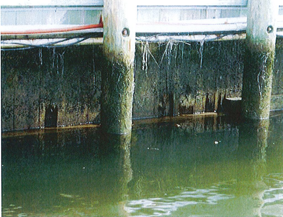
Photo 13: Deterioration of sheet piles and wales west of B Dock
