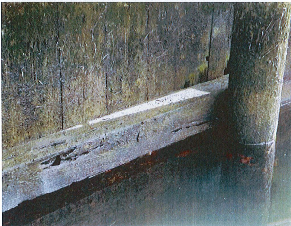
Photo 10: Wale that is east of C dock with heart rot
